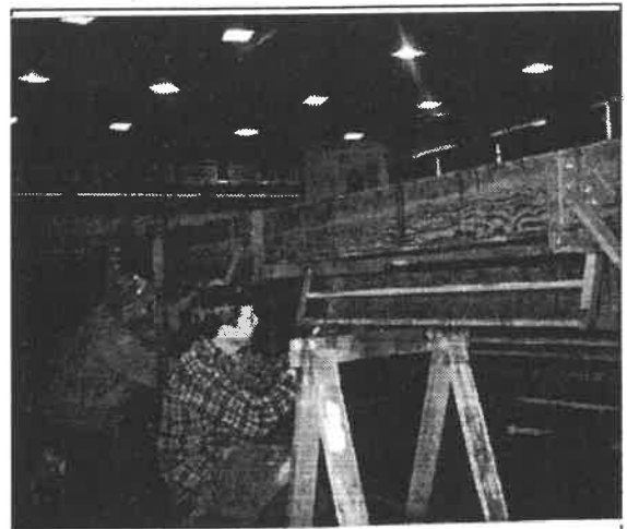
Workers repair the bleachers in the gymnasium at Somerset High School. (see article, p. 10)
